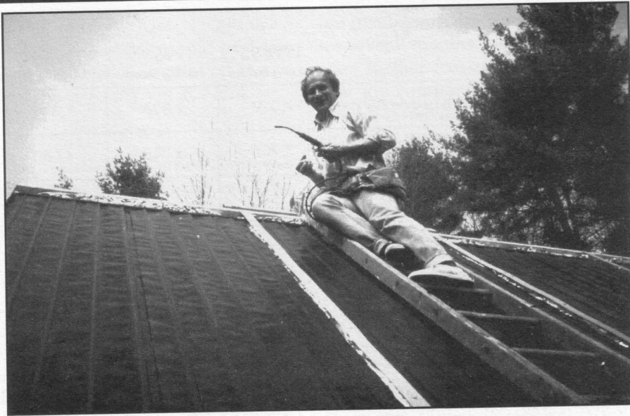
Jim Serdy, who helped design and build the active solar heating system, at work on the rooftop collectors.
